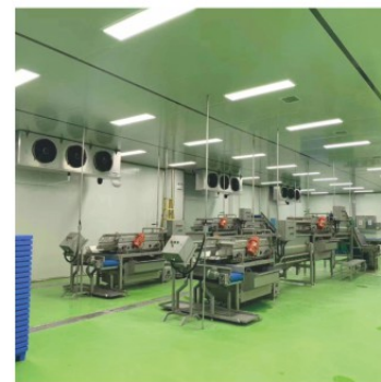
working room chilling
