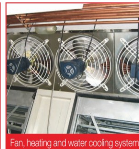
Fan, heating and water cooling system
