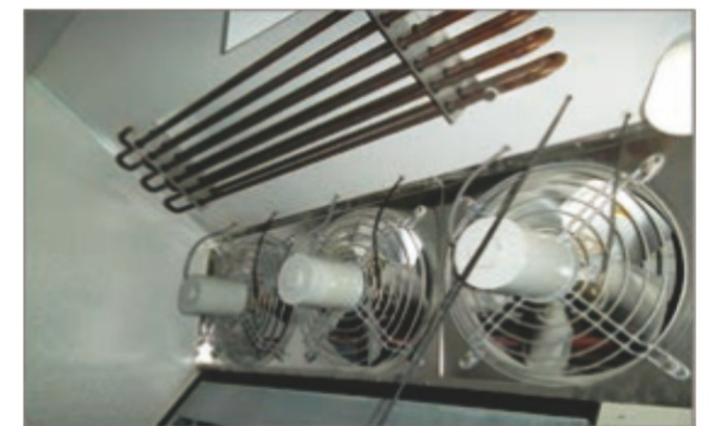
Partition fan,heating and water cooling
